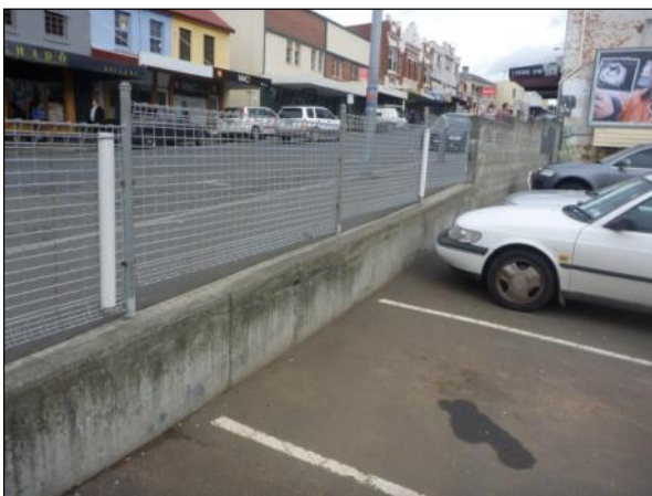
Figure 75: Retaining wall separating the car park from Elizabeth Street. Cutting varying from approximately 20cm to 1m has occurred.
