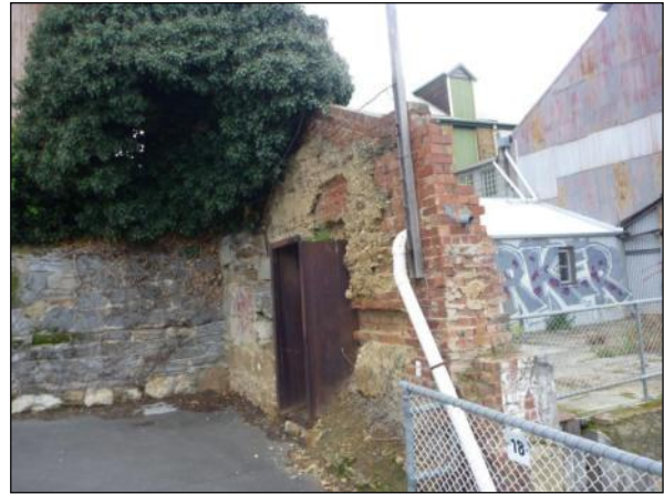
Figure 86: Ruinous brick end wall on the boundary with 37-47 Melville Street.
