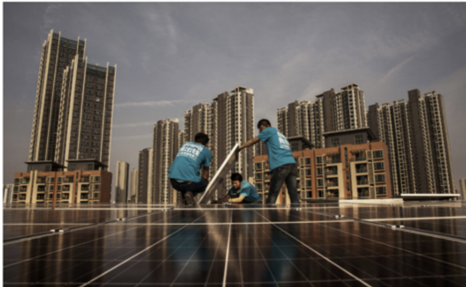
Workers from Wuhan Guangsheng Photovoltaic installed solar panels on the roof of a building in Wuhan, China, last month. China has become a defender of an ambitious climate change policy. Kevin Frayer/Getty Images
